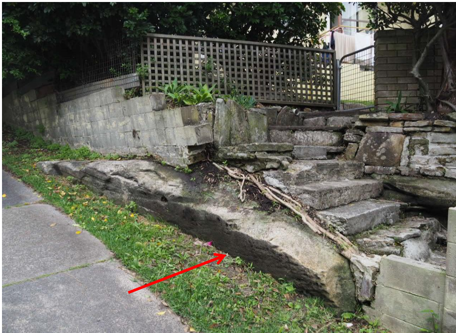
Photo 4: Sandstone bedrock and leaning boundary wall beside College Street
