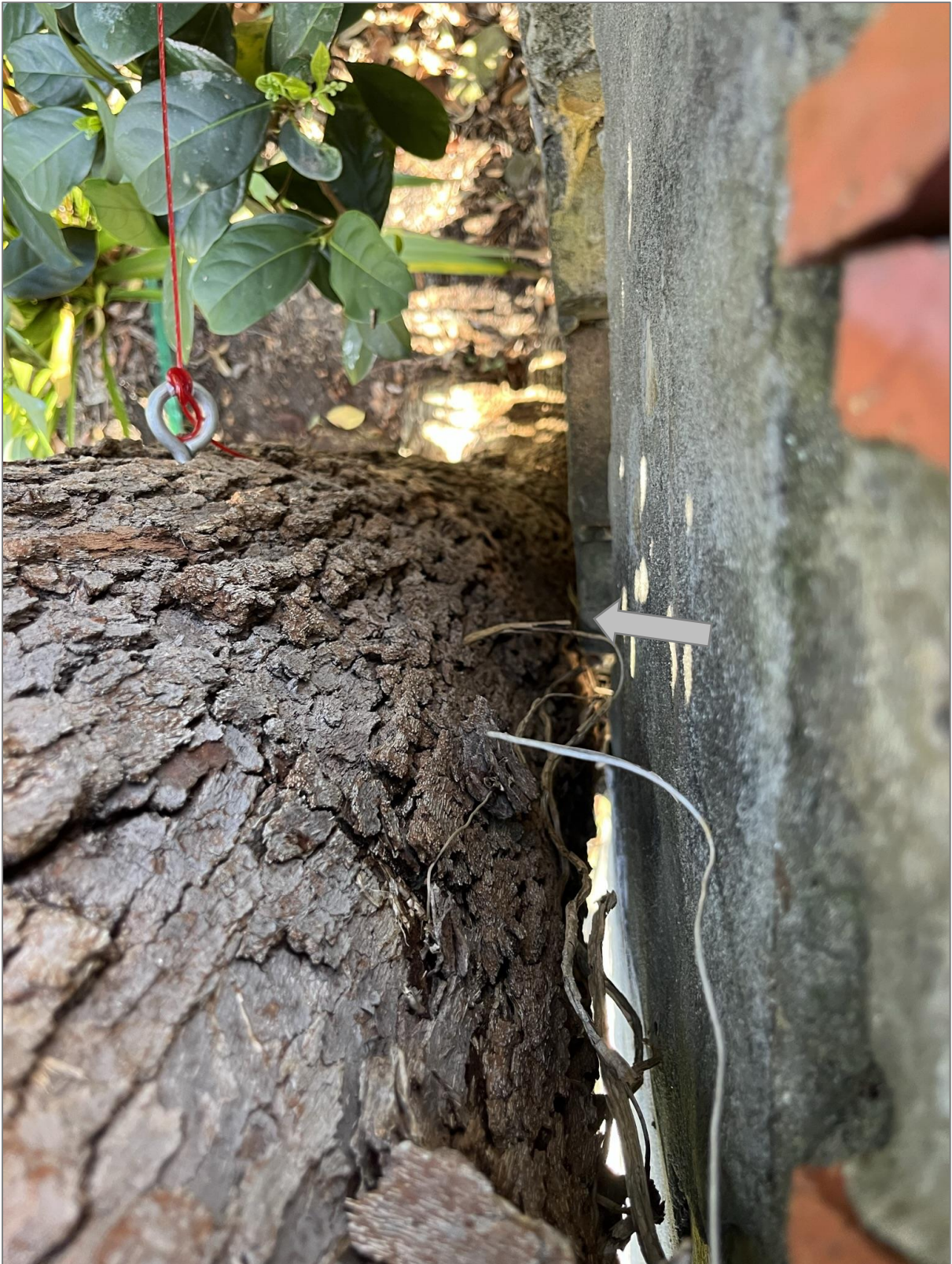
Plate 2 – Tree 1 – Arrow notes tree stem in contact with existing retaining wall.
