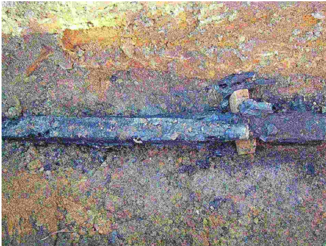
Figure 16 – Damaged bitumen encased cable
