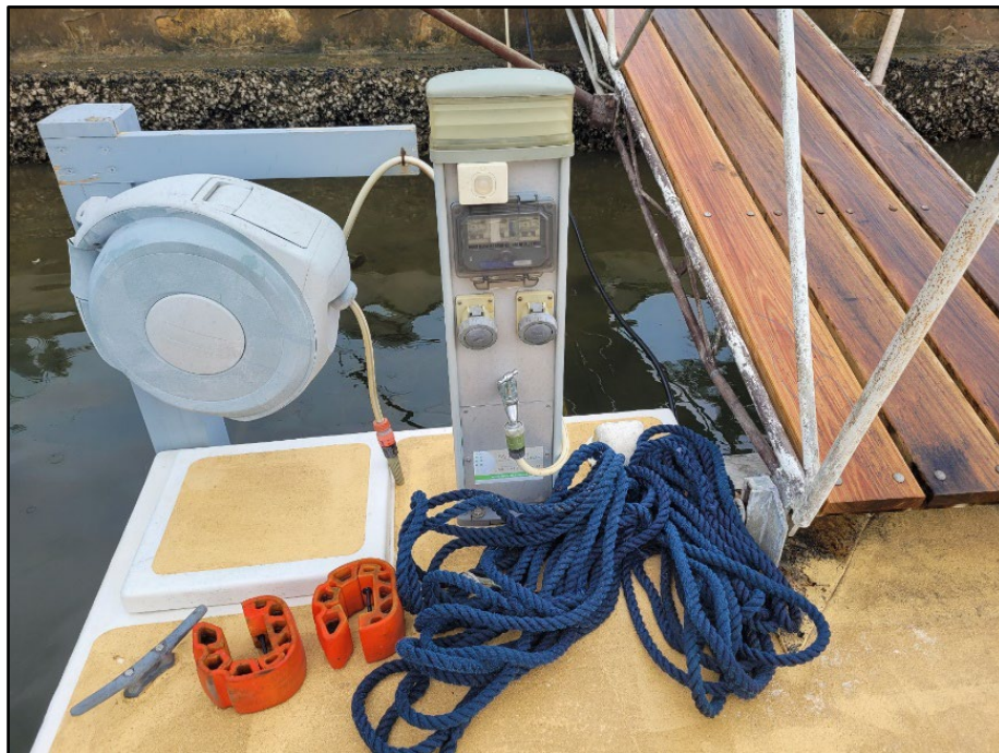
Figure 6 – existing pontoon services
