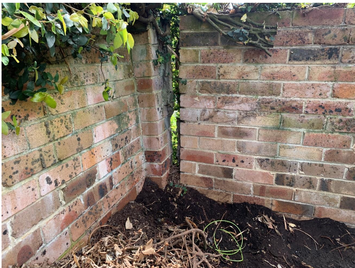
Photograph 4: Outward rotation within the western boundary wall within the rear of the site, with significant deflection and \leq 150\text{mm} separation from adjacent northern boundary wall, facing north.
