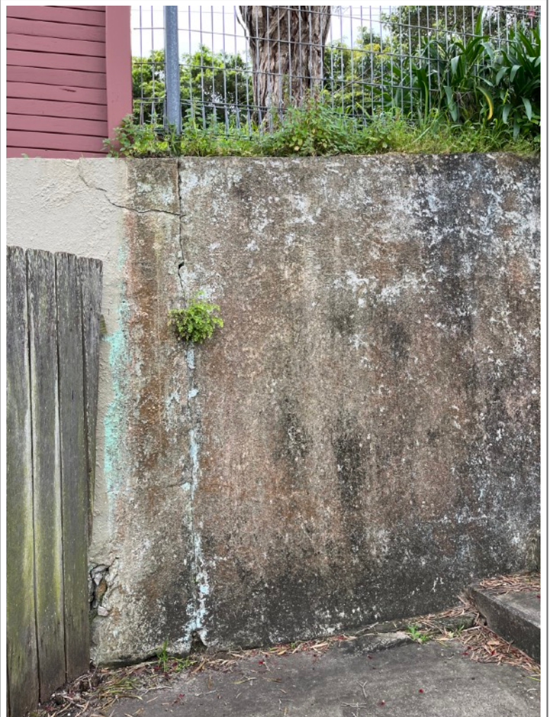
Figure 2 Shows the compromised northern boundary wall.
