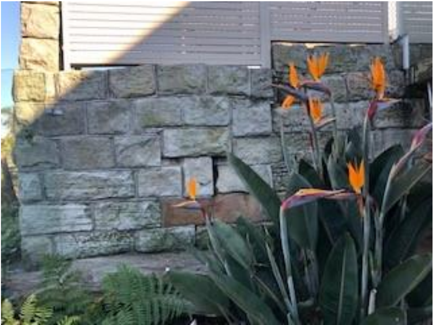
Picture 3 - retaining wall – looking to west from 45 – showing bulging and also where ground level of 45 is
