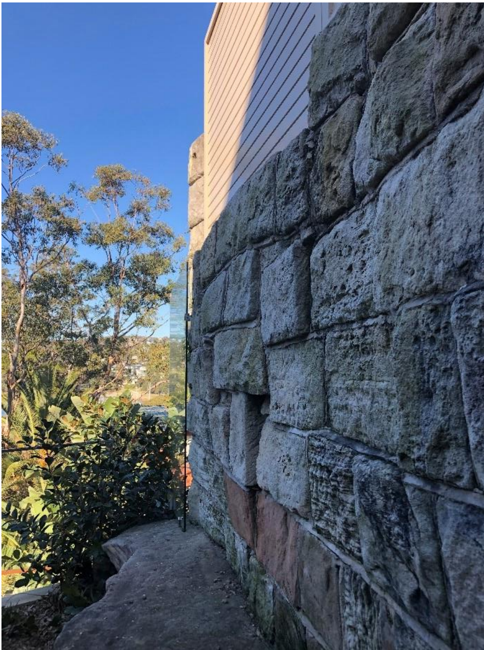
Picture 2 – retaining wall – looking to south from 45, again showing bulging and ground level of 45
