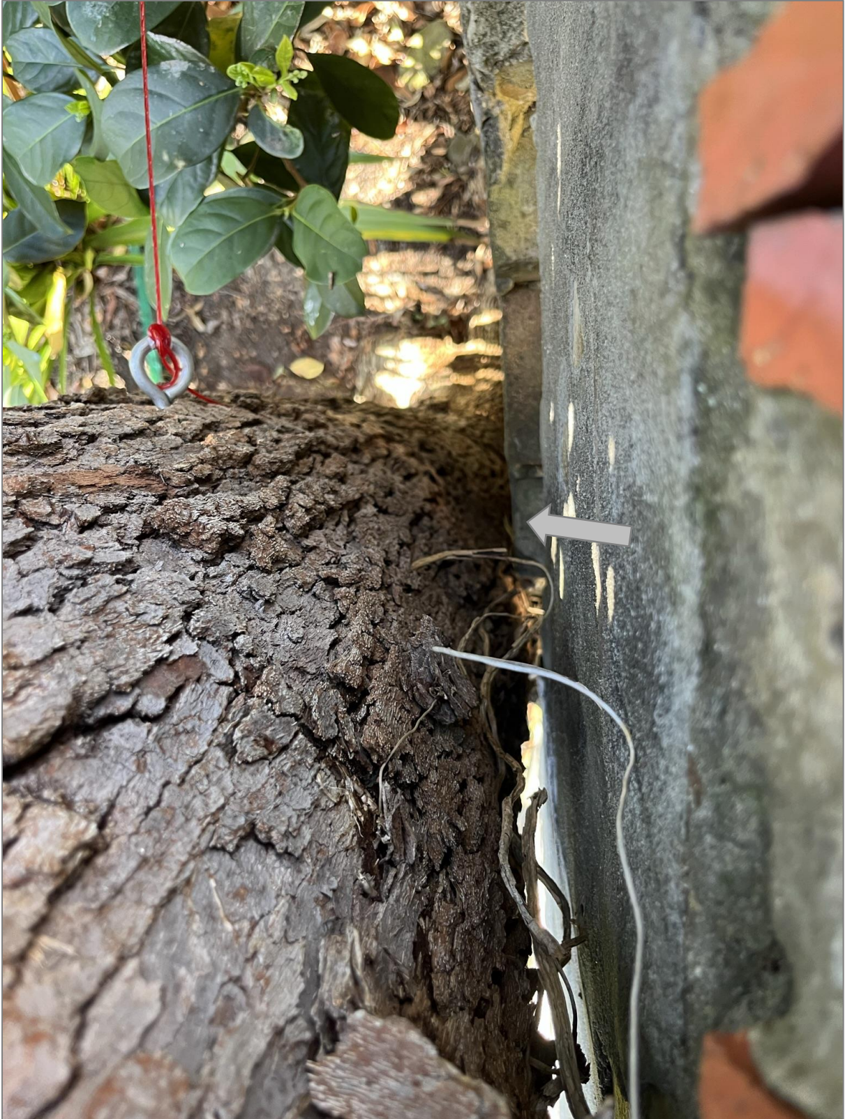
Plate 2 – Tree 1 – Arrow notes tree stem in contact with existing retaining wall, concern regarding loss of this ‘support’ and root damage during new retaining wall build leads to recommending removal of tree to facilitate new wall.
