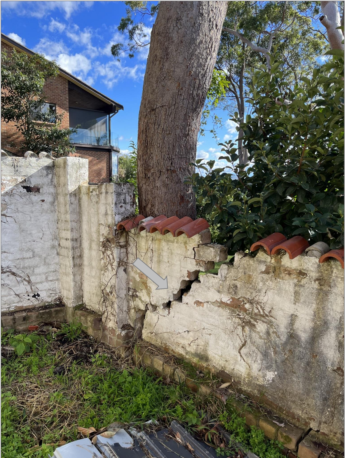
Plate 3 – Tree 1 – Arrow notes broken wall in close proximity to tree.
