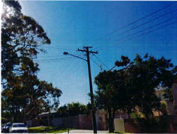
Electrical supply along Beatty Street
