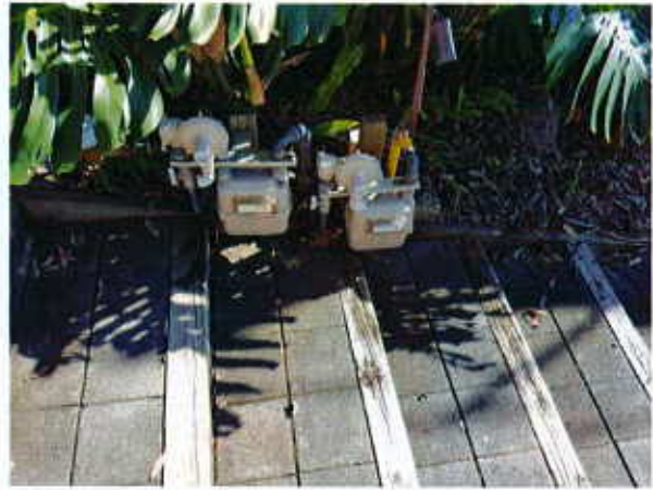
Existing gas supply point
