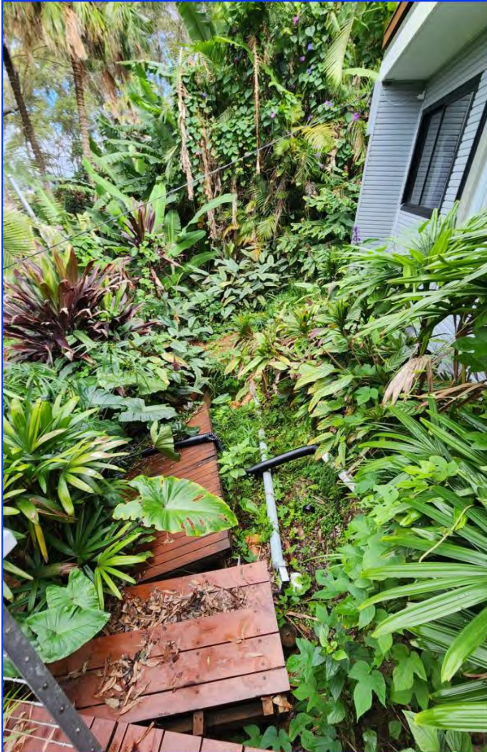
Photo 2- looking westwards showing slumped deck
