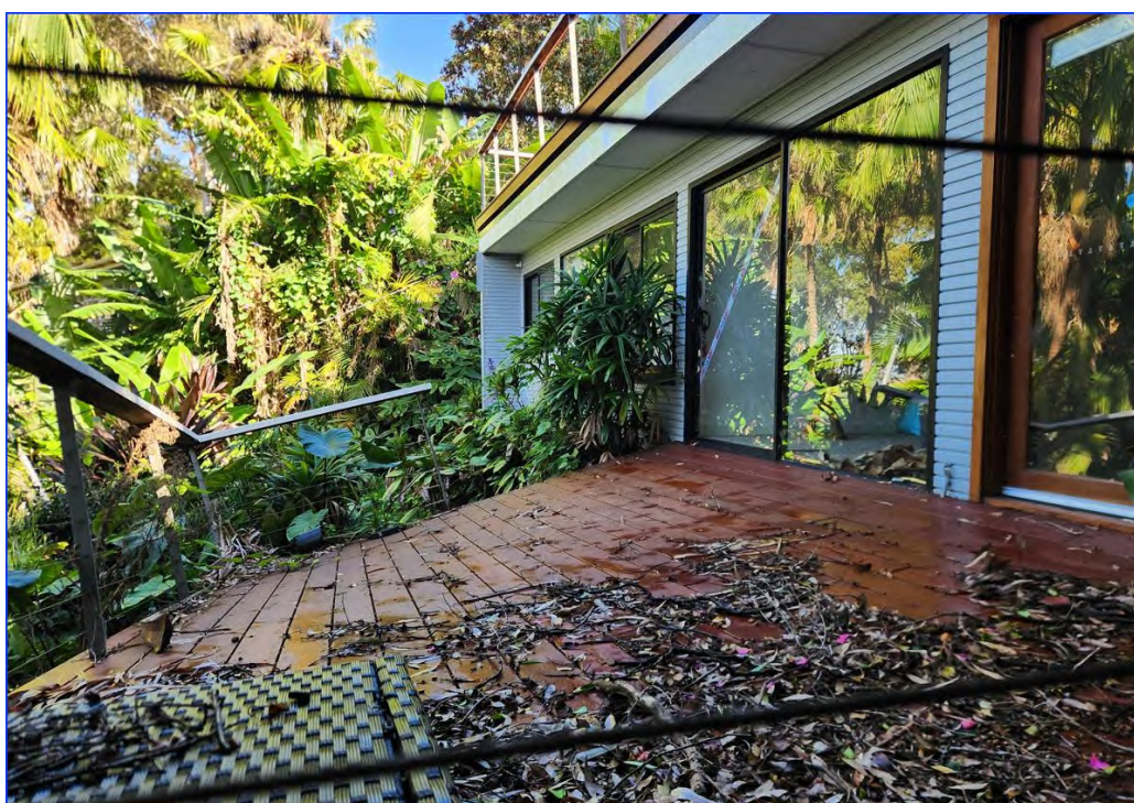
Photo 1- looking westwards showing slumped deck
