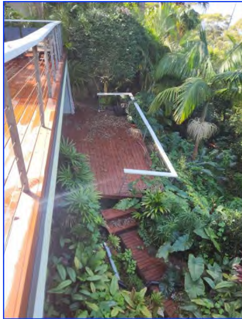
Photo 3- looking down eastwards showing damaged deck and slumped path
