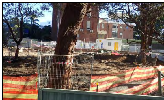
Image: Poor tree protection fencing not complying with AS 4970-2009. Image Paxton.
