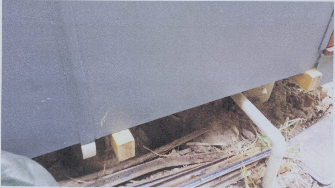
Photo 10 – View of protruding floor framing under eastern extension. These joists are to be cut back and clad.
