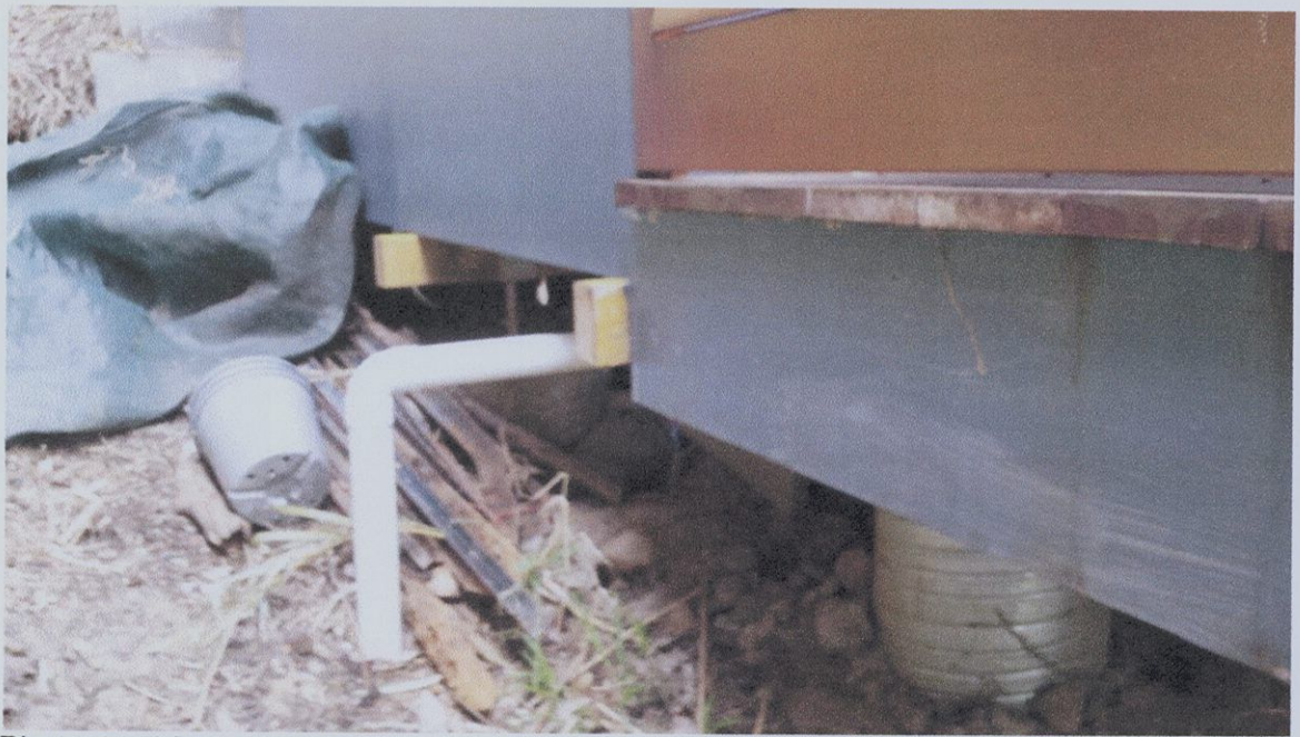
Photo 9 – View of protruding floor framing under eastern extension. These joists are to be cut back and clad.
