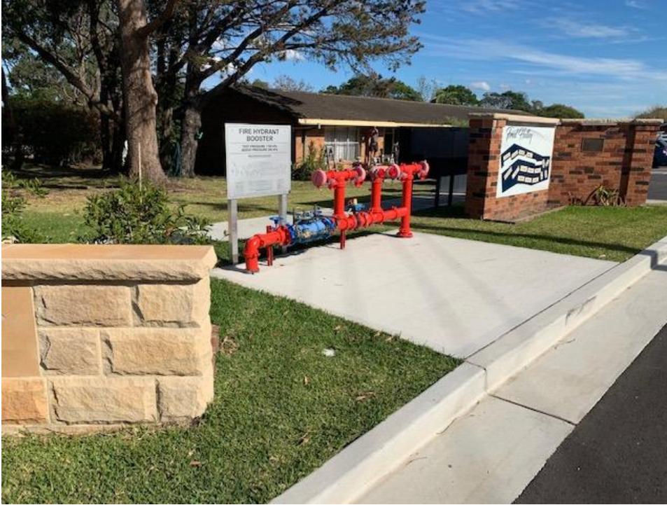
View 7 Entry where brigade valves and wall are located
