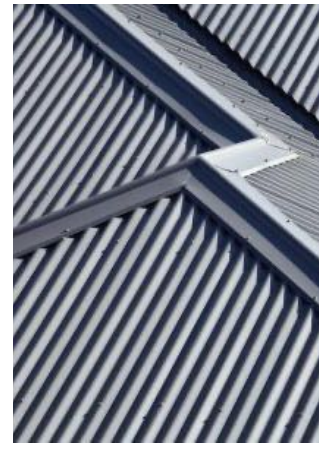
3 | Roof | Custom Orb
