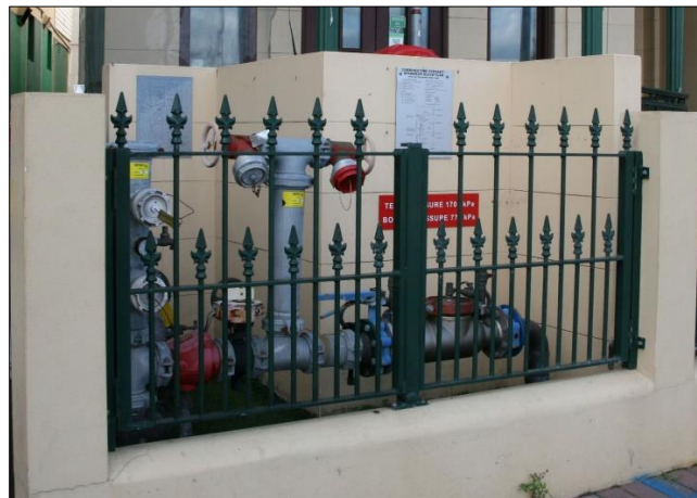
Figure 31: Location of the fire booster pump to the Street boundary of No. 50 East Esplanade.
