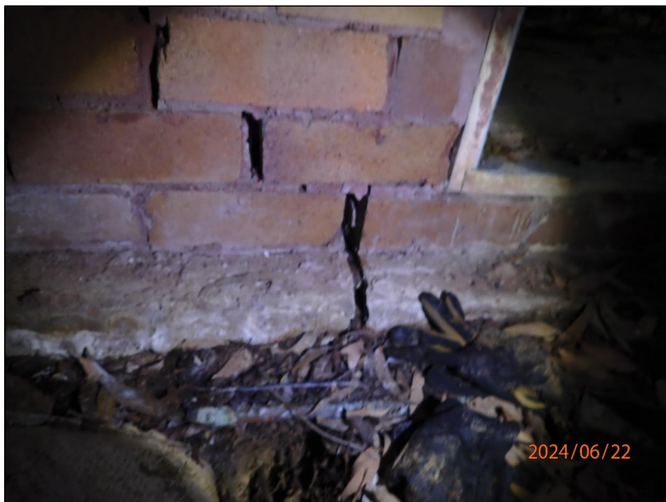
Plate 29: Cracks within brick strip footing, looking west
