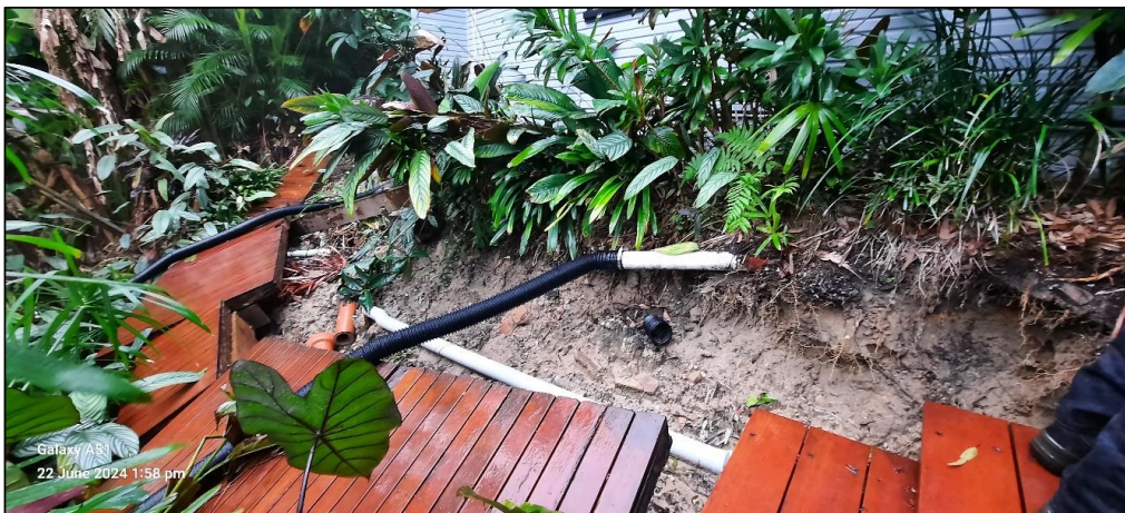
Plate 25: Landslide extending to the eastern edge of LGF level, looking west.
