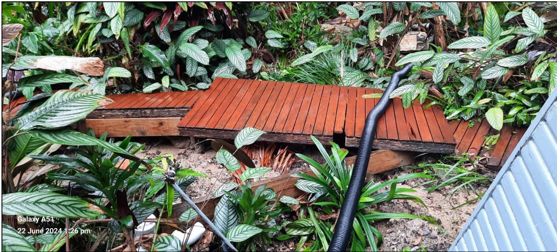
Plate 15: Timber pathway (southern half) destroyed by landslide, looking east.
