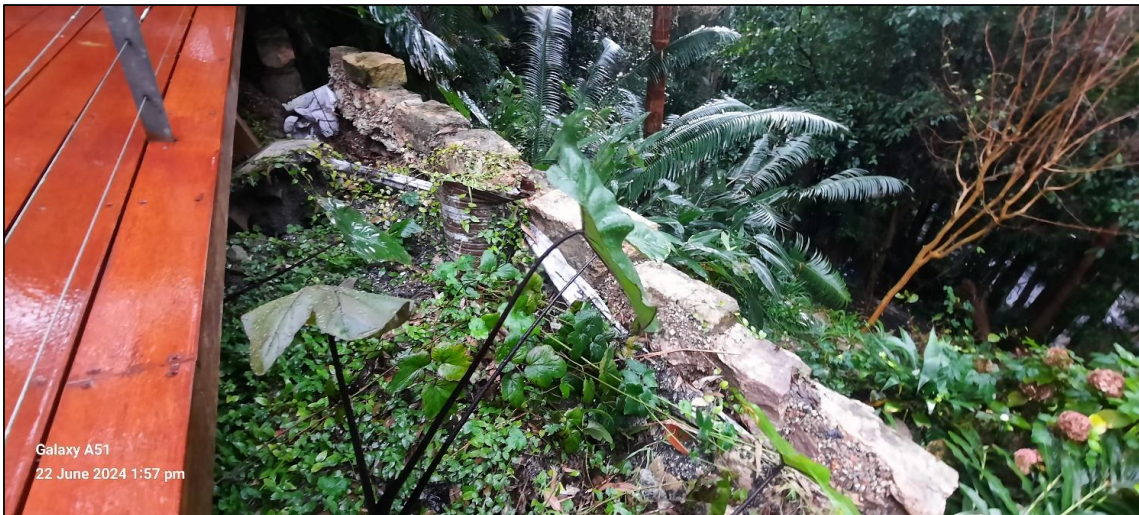
Plate 23: Completely failed stone wall, adjacent to eastern edge of timber deck at LGF level, looking north.
