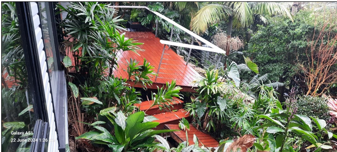
Plate 14: Timber deck (northern half) and pathway destroyed by landslide, looking north.
