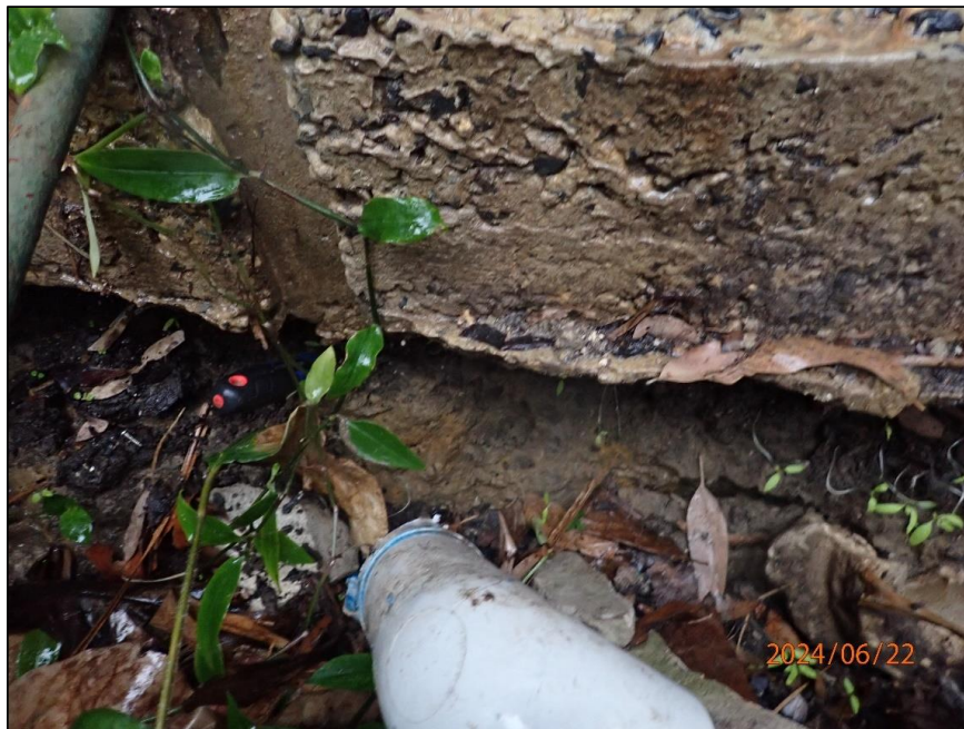
Plate 27: Undermined concrete pad of brick strip footing supporting LGF level, looking north-west.
