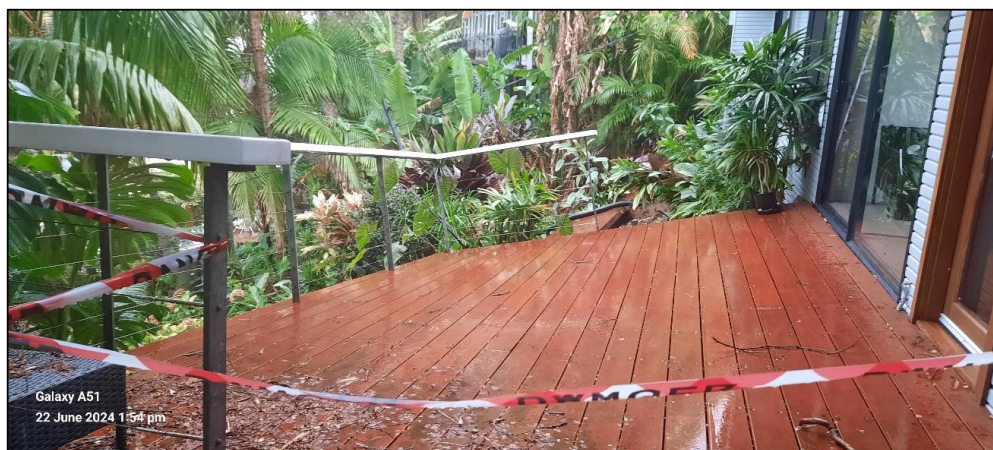
Plate 19: Displaced timber deck at LGF level, looking south.
