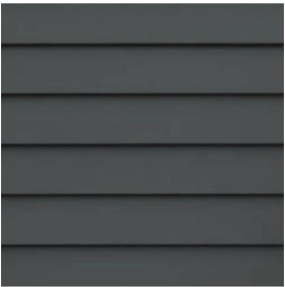
2. Weatherboard Cladding - "Dulux Western Myall" Colour
