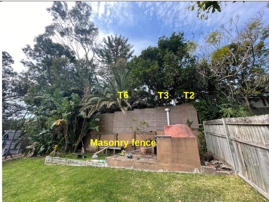
Photo 2: Looking East from within the site towards tree 2, 3 and 6 (located within the adjoining property). The existing boundary masonry fence appears to be restricting root growth into the subject site.
