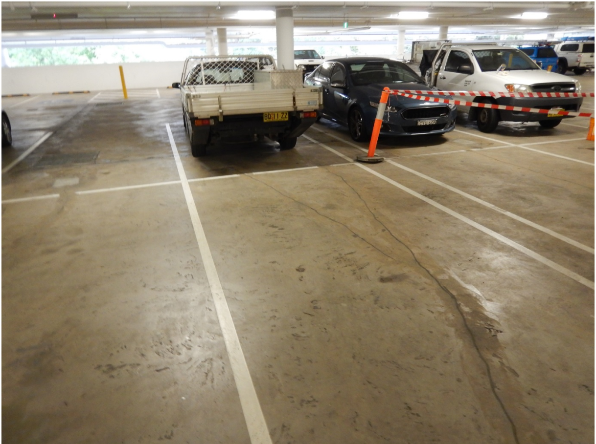
Photograph 3: Sealed Post Tension Cracks
