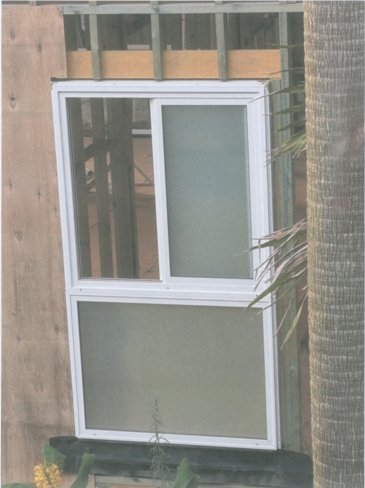
FIG 6: W6 shows the open window which is not compliant with condition 2(a)(i) or (ii). This window is located opposite bedrooms of 948.
