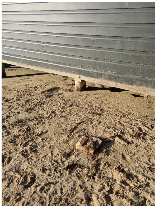
Figure 11 – Photo showing position of exposed concrete pile from old boatshed
