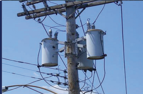
Pole Transformer (PT)
