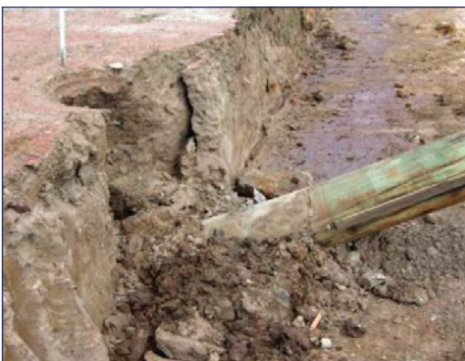
Excavation causing pole collapse
