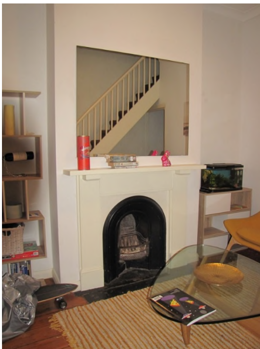
Figure 19: Original fireplace with cast iron insert and plan joinery surround – to be retained in front room.
