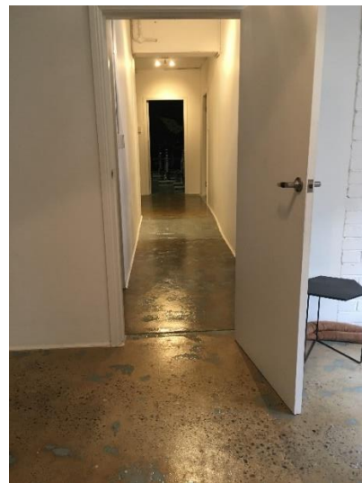
5.4.5d – No directional exit signage above doorway
