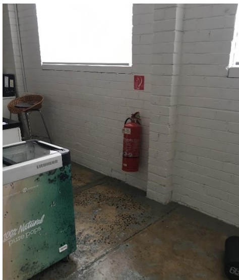
Figure 5.4.3 – Portable fire extinguisher installed
