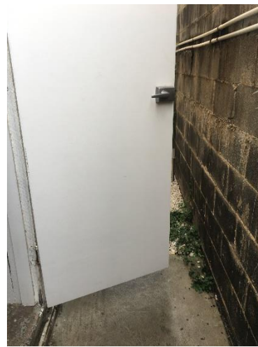
Figure 5.3.8b – Door impeding path of egress
