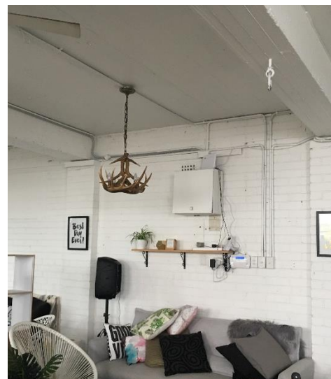
Figure 5.3.3b – View of electrical meters / distribution boards 2
