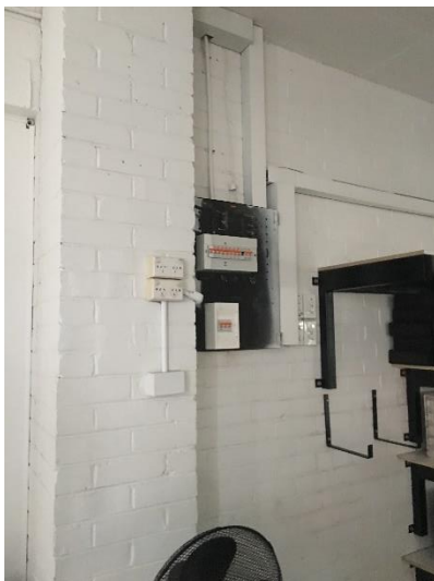
Figure 5.3.3a – View of electrical meters / distribution boards 1
